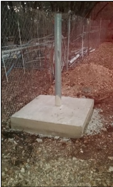
Tower Dead Man Cable Support x's 3 3'6" x 3'6" x 3' with Sched 40 Pipe
