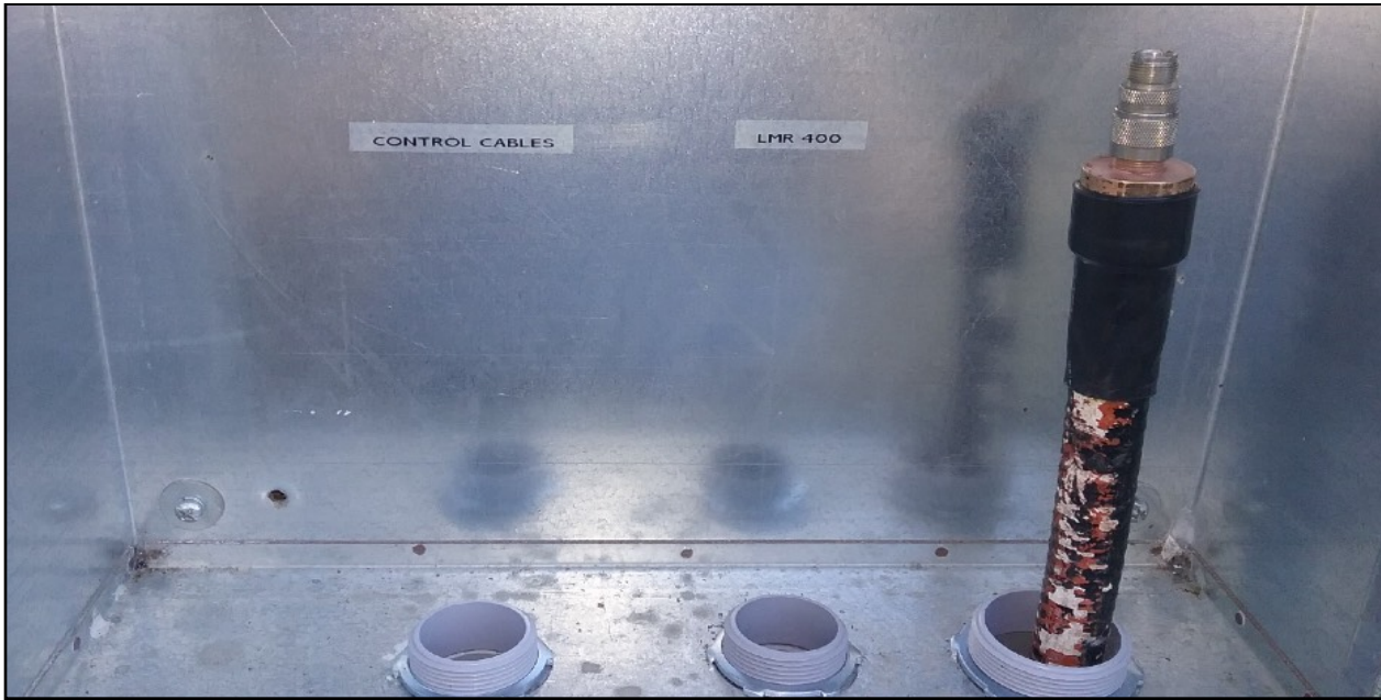
Inside the Enclosure Panel Mounted at base of tower with Conduit Feeds for 7/8" Hard Line, LMR-400 runs, and Control Cables for Rotors, Antenna Switch relays, and Power over Ethernet, Mesh Nodes etc.
